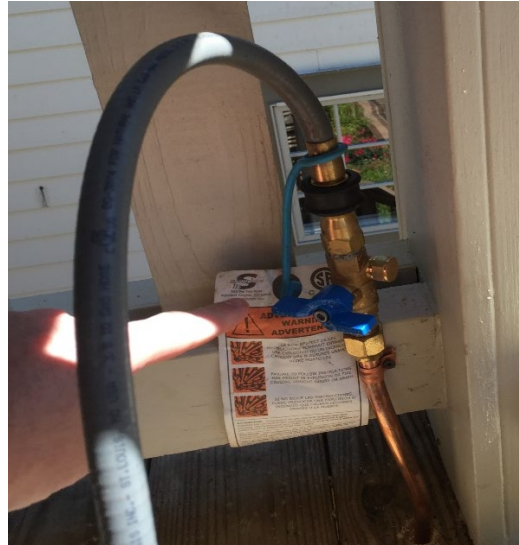
Blue valve closed; no gas flowing.
