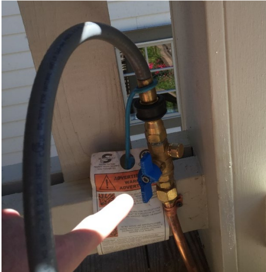
Blue valve open; gas is flowing.
