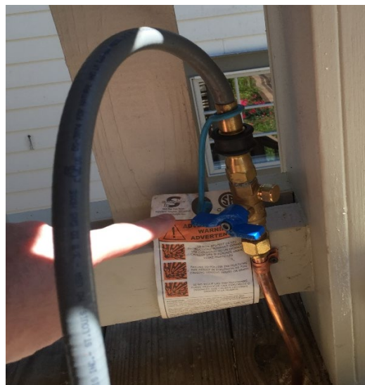
Blue valve closed; no gas flowing.
