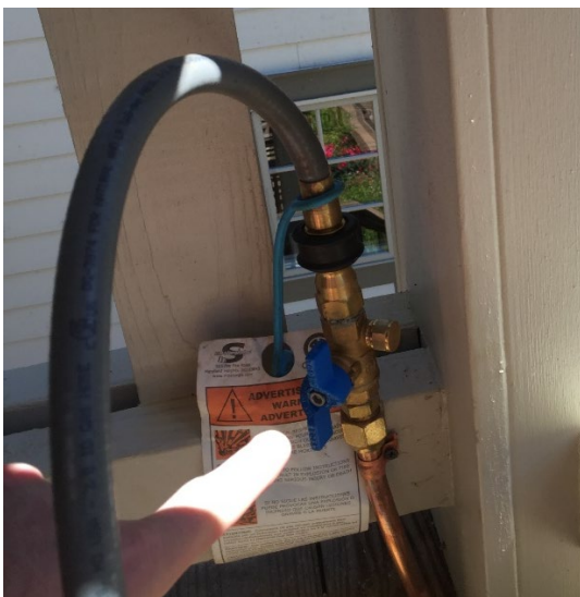
Blue valve open; gas is flowing.
