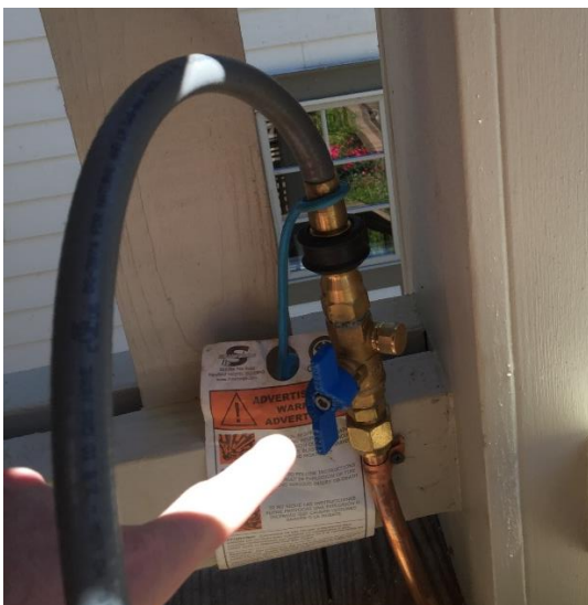
Blue valve open; gas is flowing.
