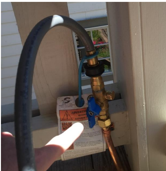
Blue valve open; gas is flowing.
