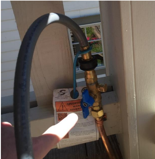
Blue valve open; gas is flowing.
