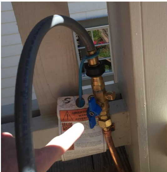
Blue valve open; gas is flowing.
