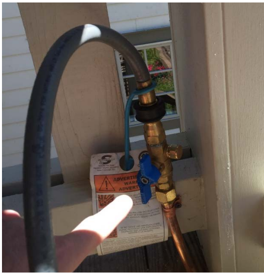
Blue valve open; gas is flowing.
