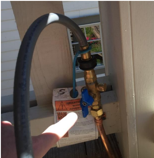
Blue valve open; gas is flowing.
